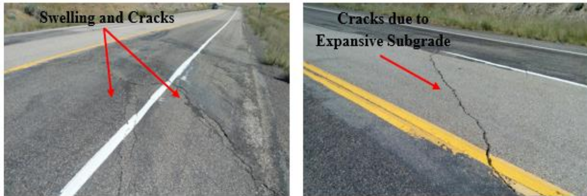
Figure 1.3 Pavement Distresses on US 95 pavement section (MP 16.7 to MP 18.5) due to expansive subgrade
